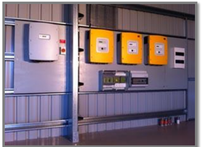
Figure 4 Off Grid Solar Management Hub
