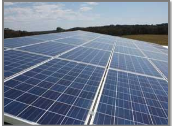
Figure 3 Rooftop Solar Panels
