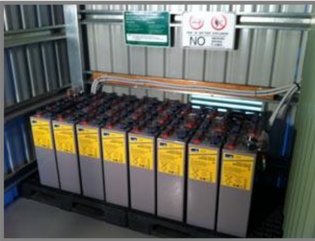
Figure 2 Solar Battery Bank
